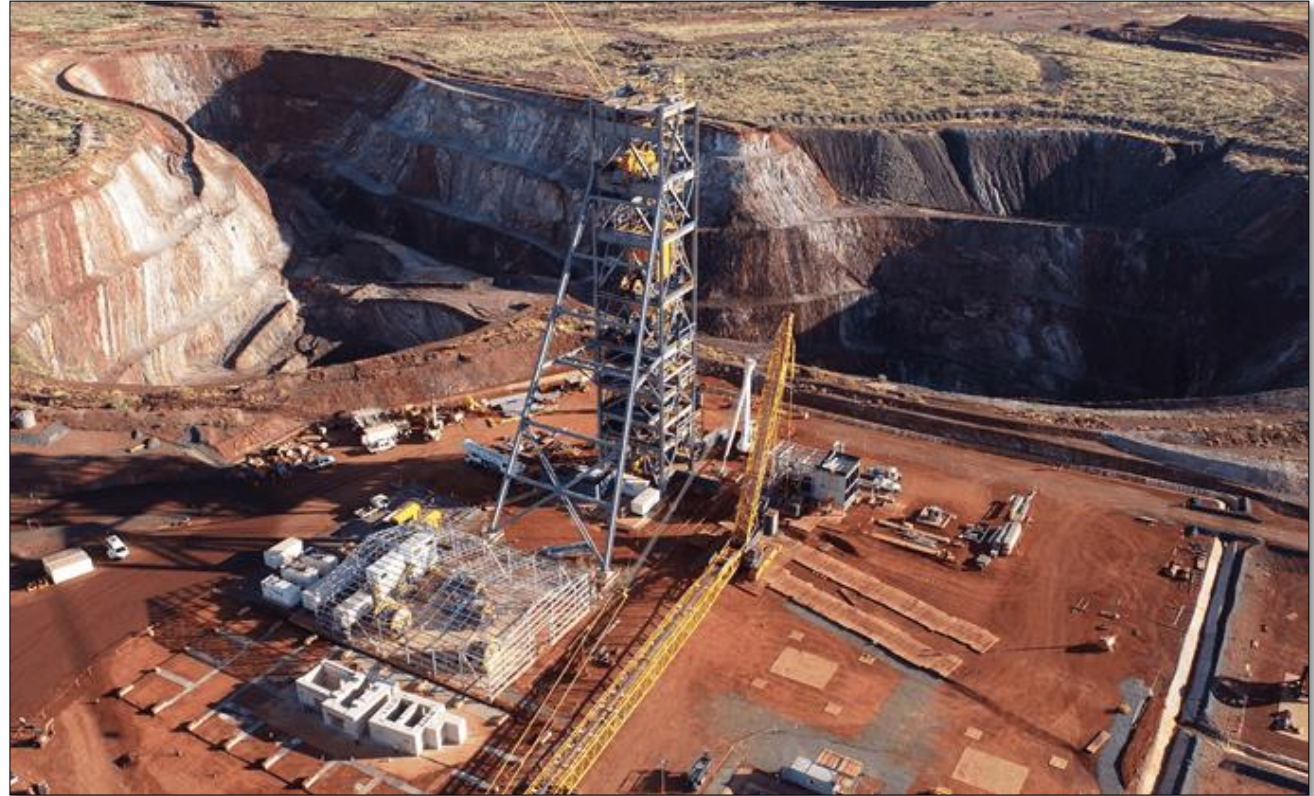
TE2 Headframe – Newmont's Tanami Gold Operations
